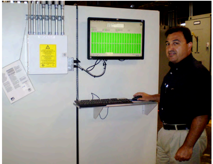
Joe Montemayor, Southern Union Data Center Operations Manager, reviews the Cellwatch system monitoring UPS batteries. No failures have been detected.
